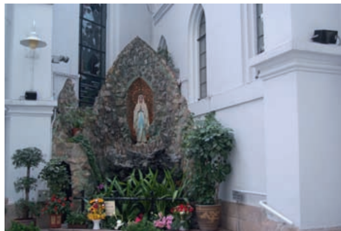
The Technomad installation outside the cathedral
